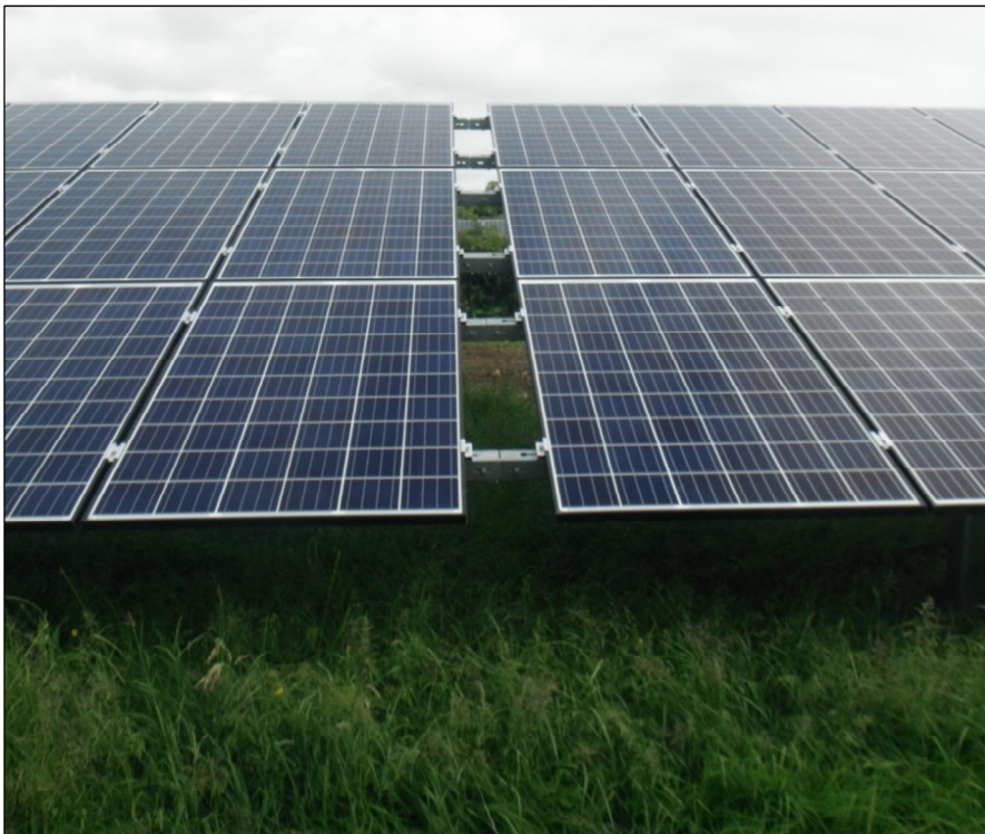
Figure 5.1 Photo of solar panels (front elevation)
