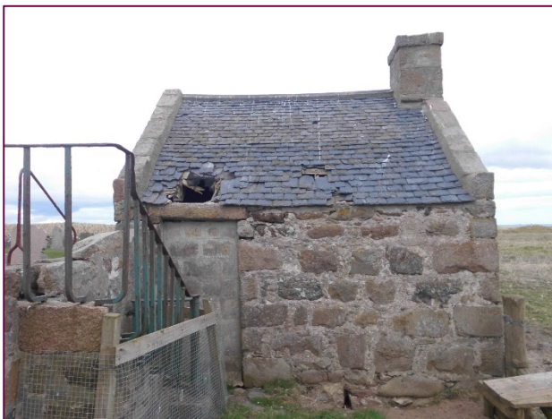
Photo 15: Derelict building of St Fergus Church offers moderate bat roosting potential.
